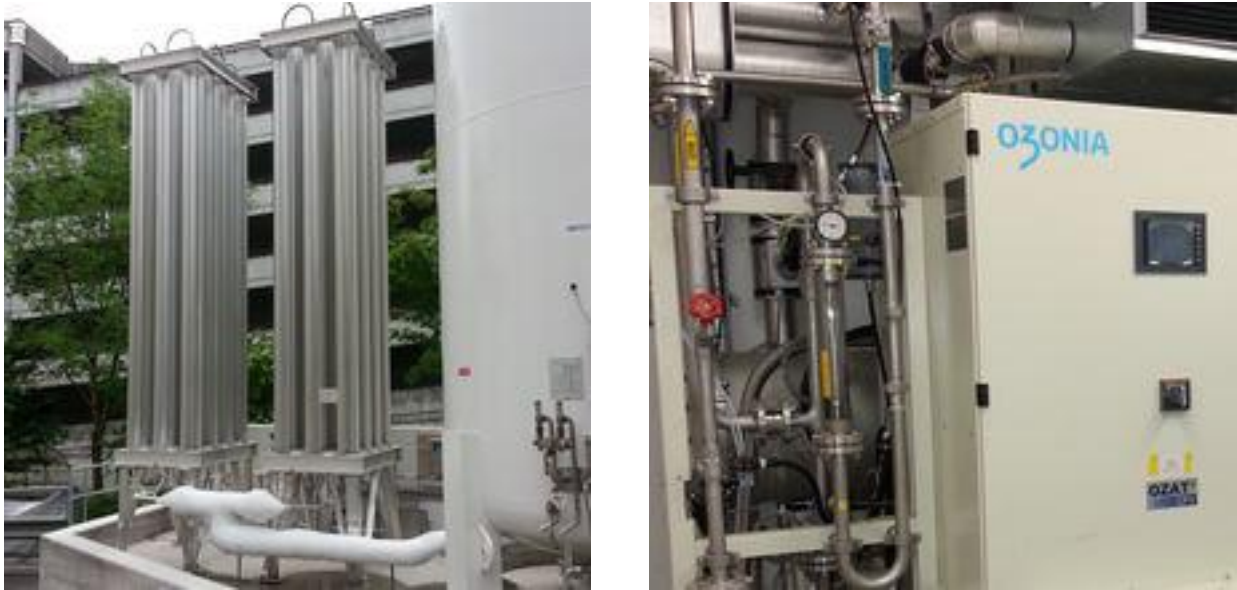
Figure 5-3: Oxygen tank with evaporator, ozone generator
